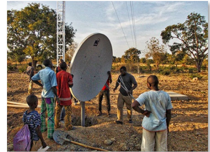
Figure 9: AMN base station in Benin. Source: VLN
